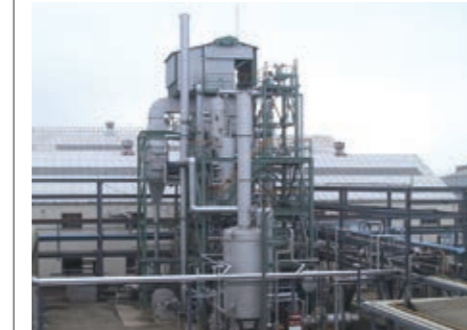
HiCOT Demonstration Plant (H 2 :1,200 Nm³/Hr)
