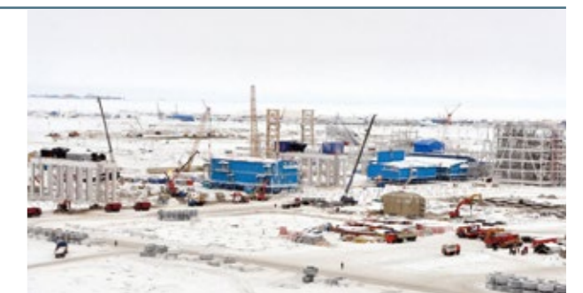
Yamal LNG construction site overview: Construction work continues all through the year
