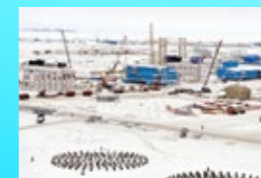
2014 Order awarded for Yamal LNG Project in Russia
