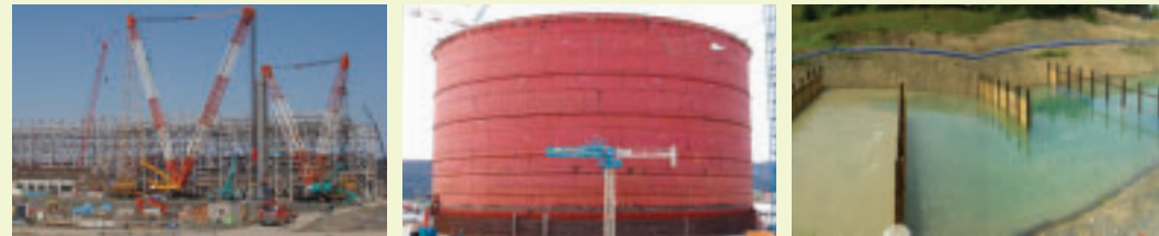
(Left) Work is proceeding on the main pipe racks. (Center) Construction of the LNG storage tank (Right) Storage pond for treating effluents
