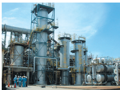
Ultra-deep desulfurization (gas oil) plant for Taiyo Oil Co., Ltd.
