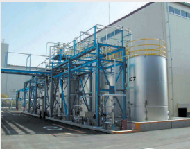
Lube Oil Blending Plant (Sanwa Kasei Industrial Corporation)
