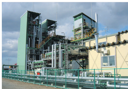
The GTL pilot plant at Yufutsu.
