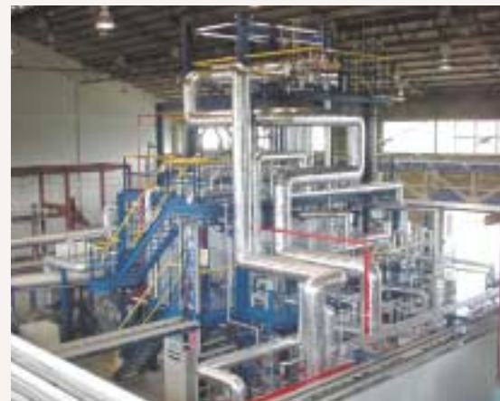
A view of the HiCOT demonstration plant
