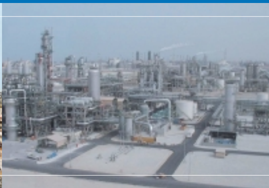
Ethylene Glycol Plant (450,000 t/y) Eastern Petrochemical Company (SHARQ) (Al-Jubail, The Kingdom of Saudi Arabia)
